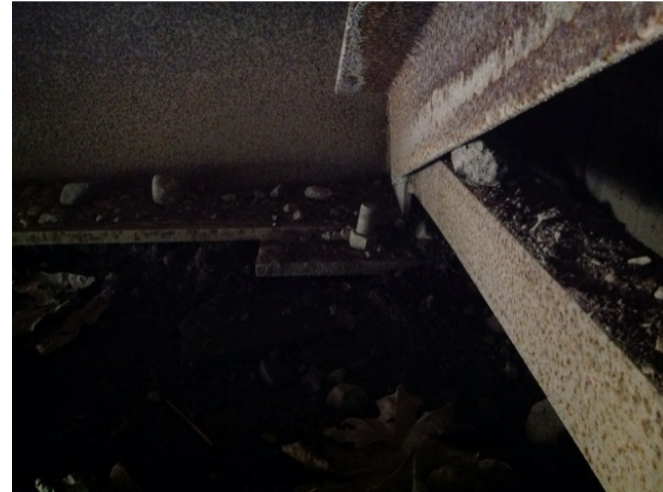
right downstream bearing bolt
